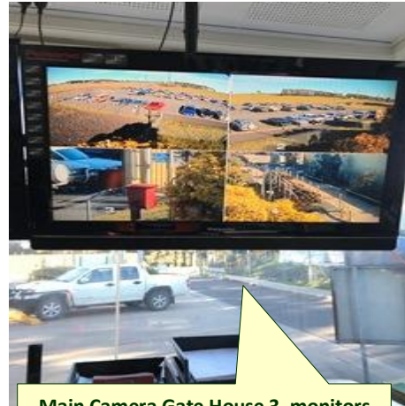
Main Camera Gate House 3, monitors all trucks entering and leaving site
