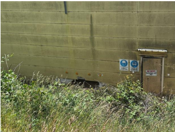
7. The site inspection identified a door was open on the dry mill southern boundary thereby limiting effective noise attenuation.
